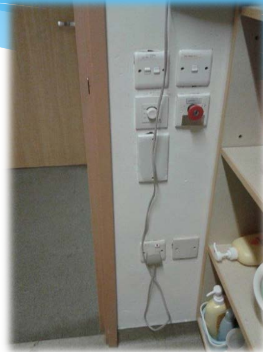
Emergency call bells in bedroom and toilets
